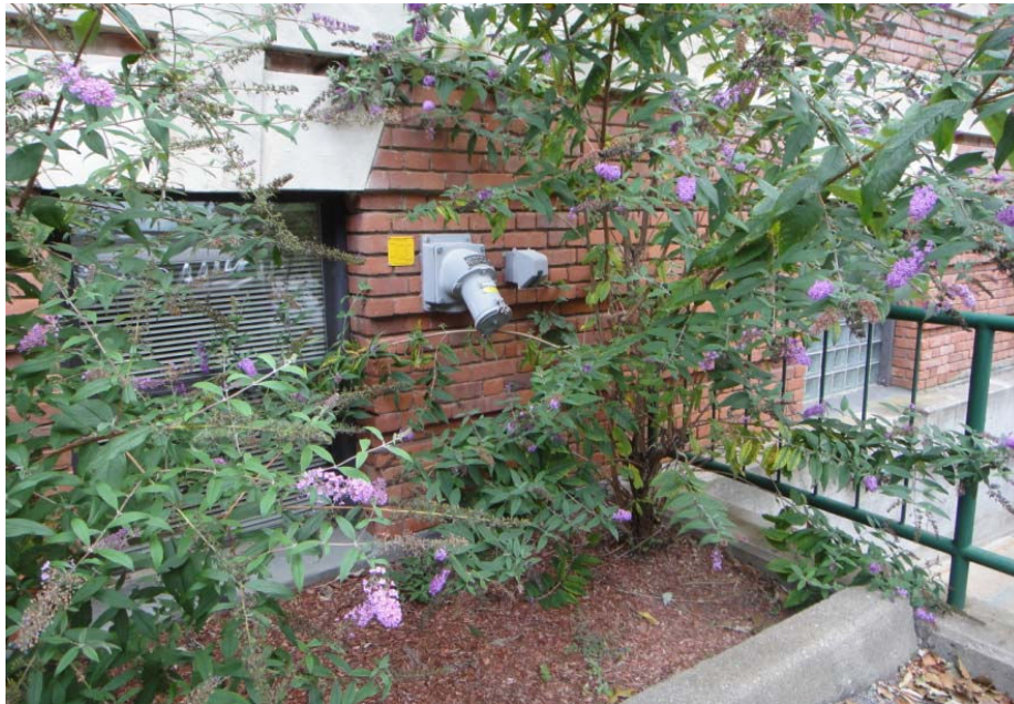
Nextel generator receptacle on east side of Municipal Building
