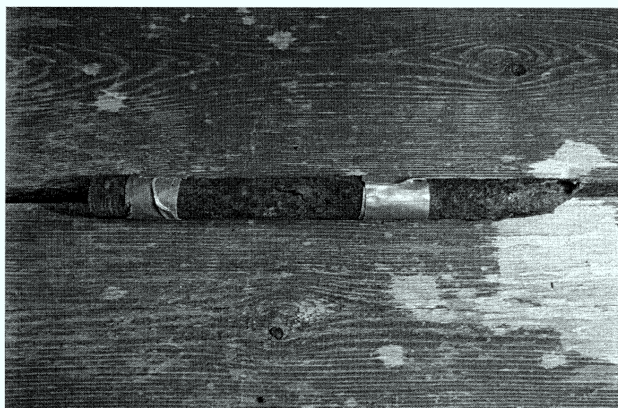
Figure 3 – Galvanized steel water service pipe with corrosion hole in center of picture, encountered during the Harmon Water Main Replacement Project area in the Village, 2005
