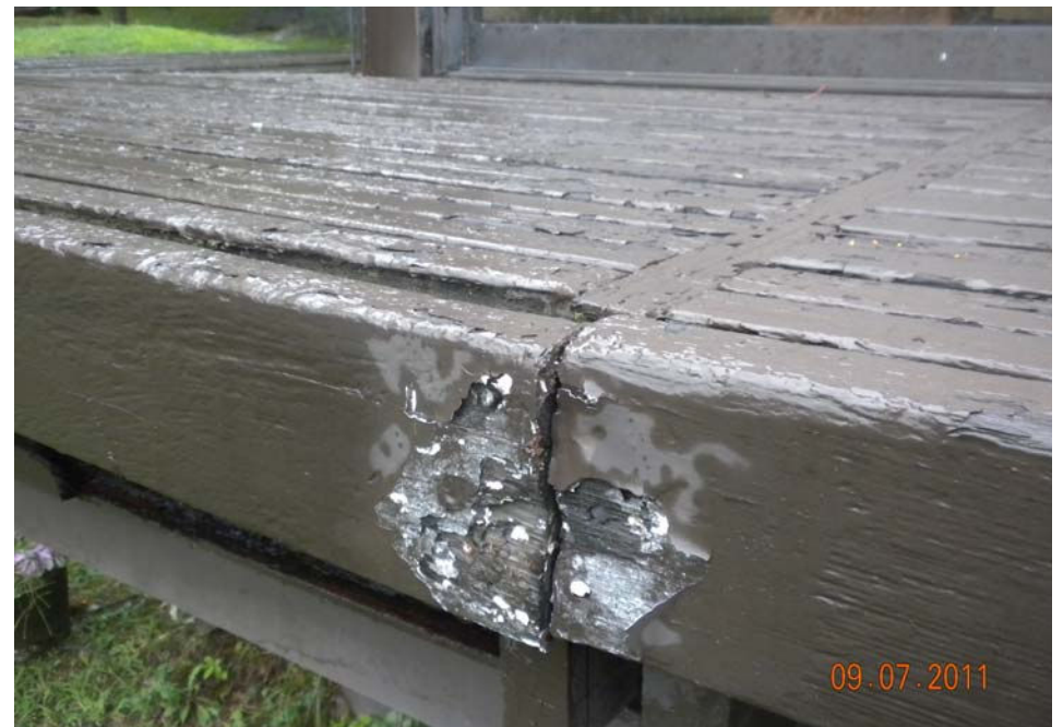
Wood rot at perimeter deck of main house
