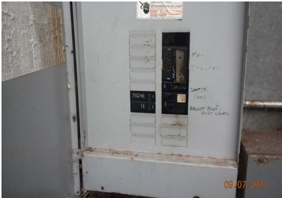
Main electrical service panel
