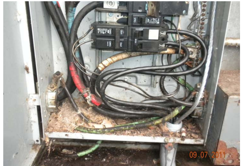
Nest in bottom of main electrical panel
