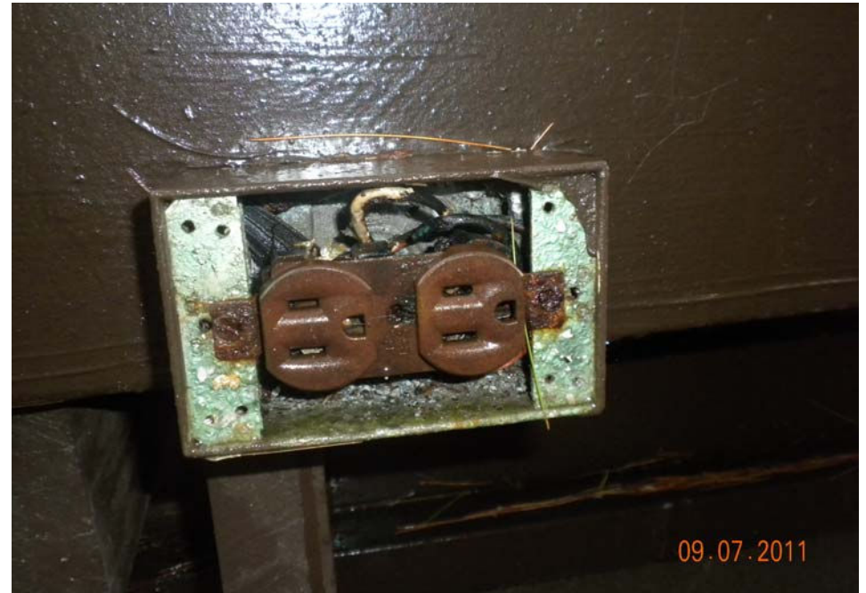
replace exterior outlets with GFCI weatherproof type
