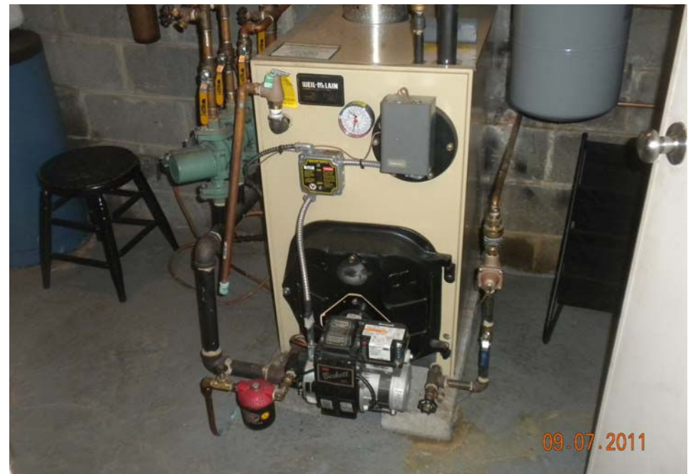
Boiler for main house
