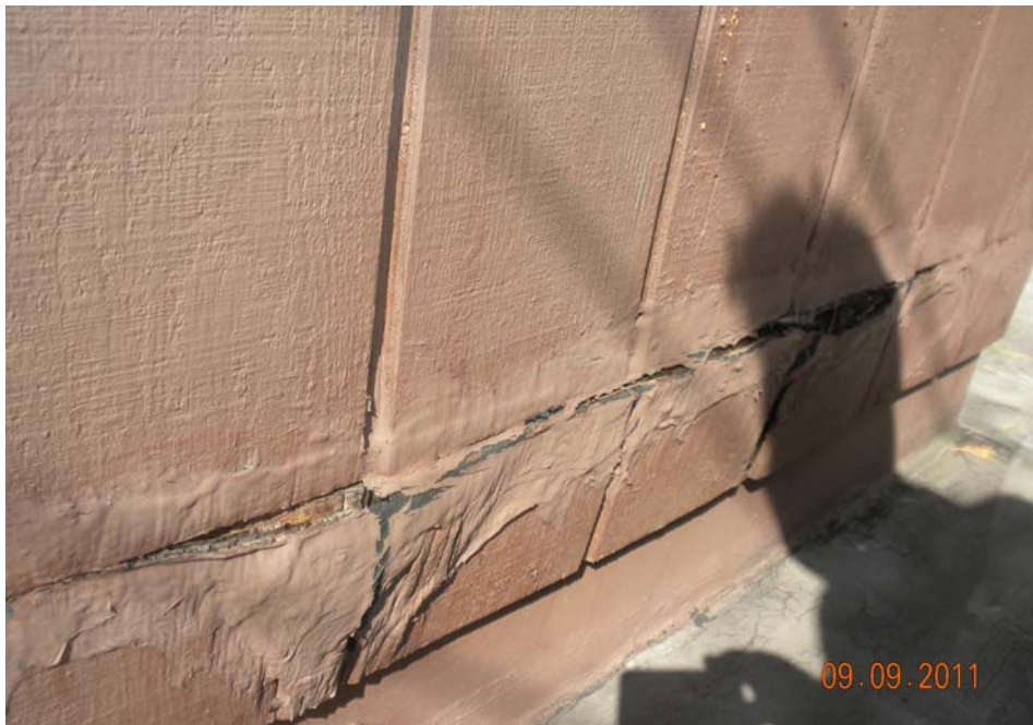
Rotted siding at main house chimney
