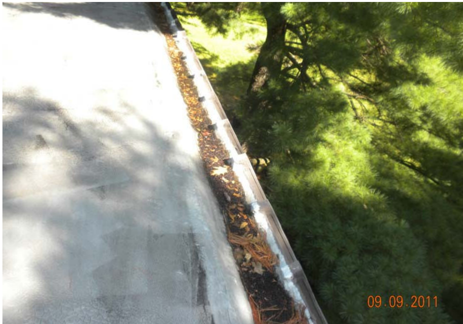
Clogged built-in roof gutters at main house
