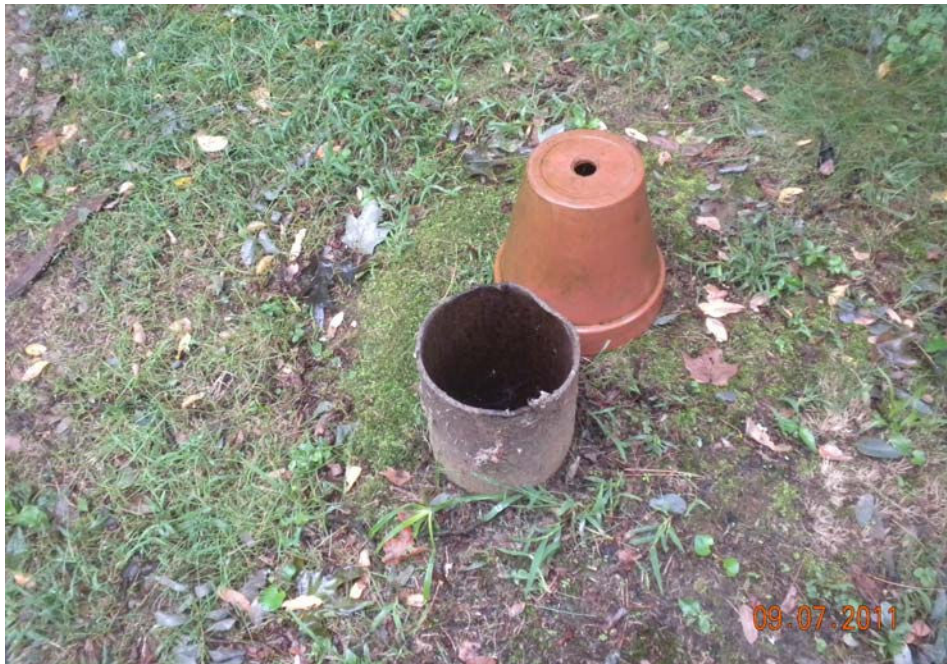
Open well casing needs to be sealed
