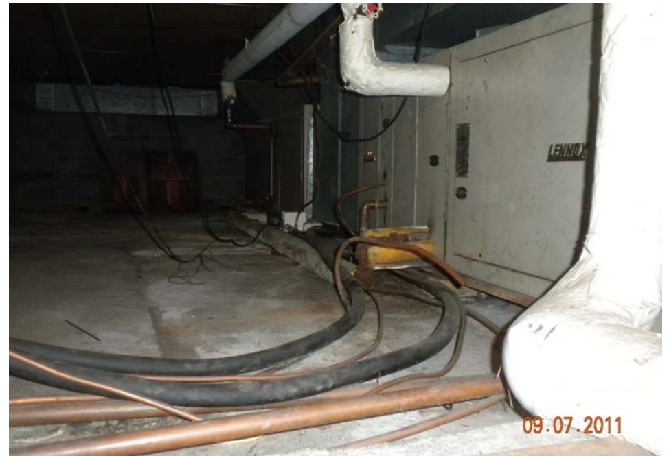
Air handlers at main house are aged
