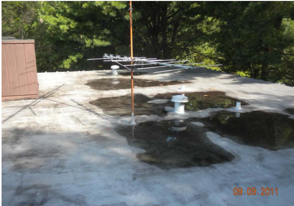
Ponding water on roof
