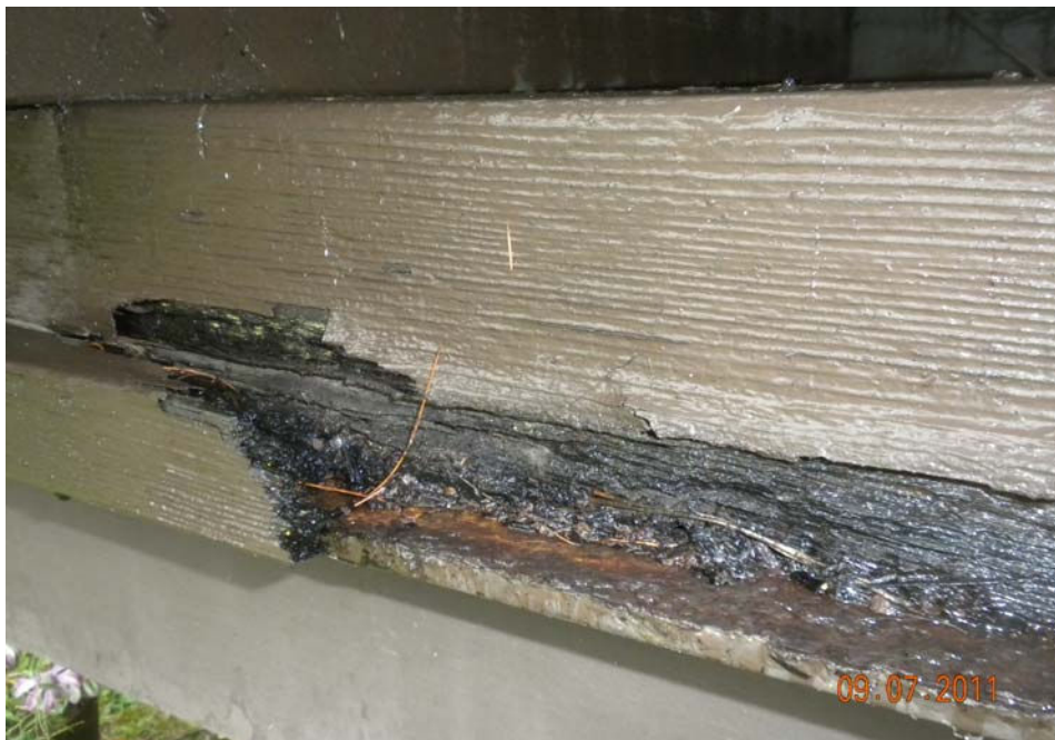
Wood rot at perimeter deck of main house
