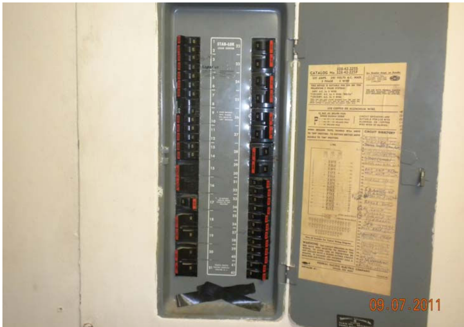
Federal Pacific electrical panel at main house
