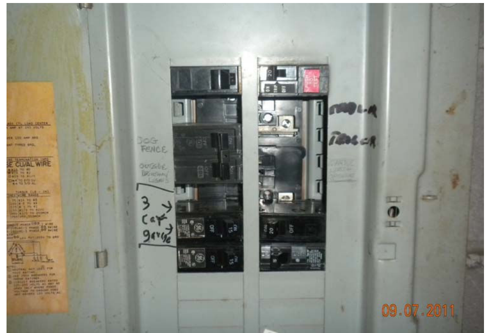
100 amp service panel in garage
