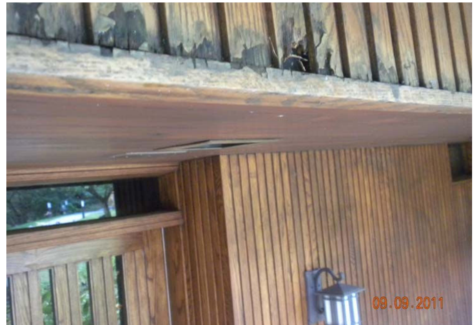
Wood Rot above entry door at main house
