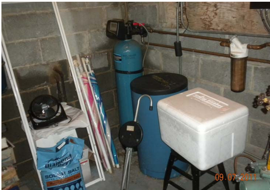
Water softener at main house
