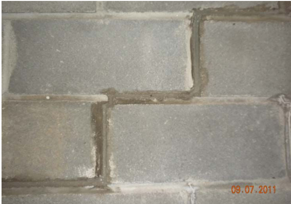
Foundation cracking at west wall of garage
