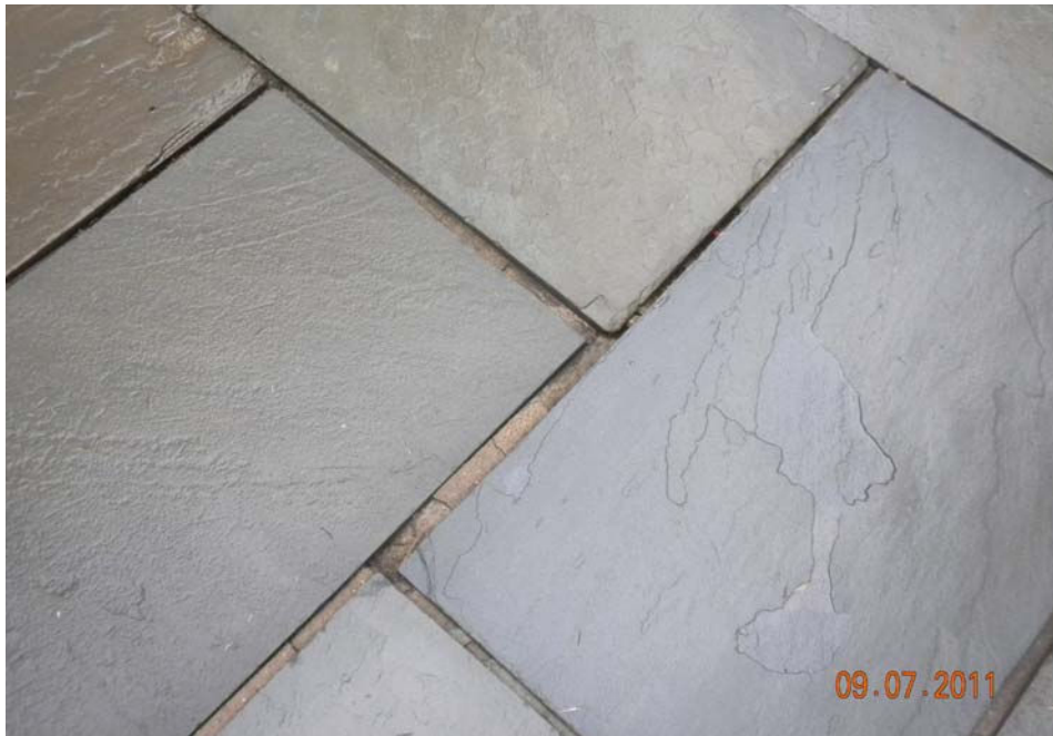
Pointing maintenance is recommended at walk and patio of main house
