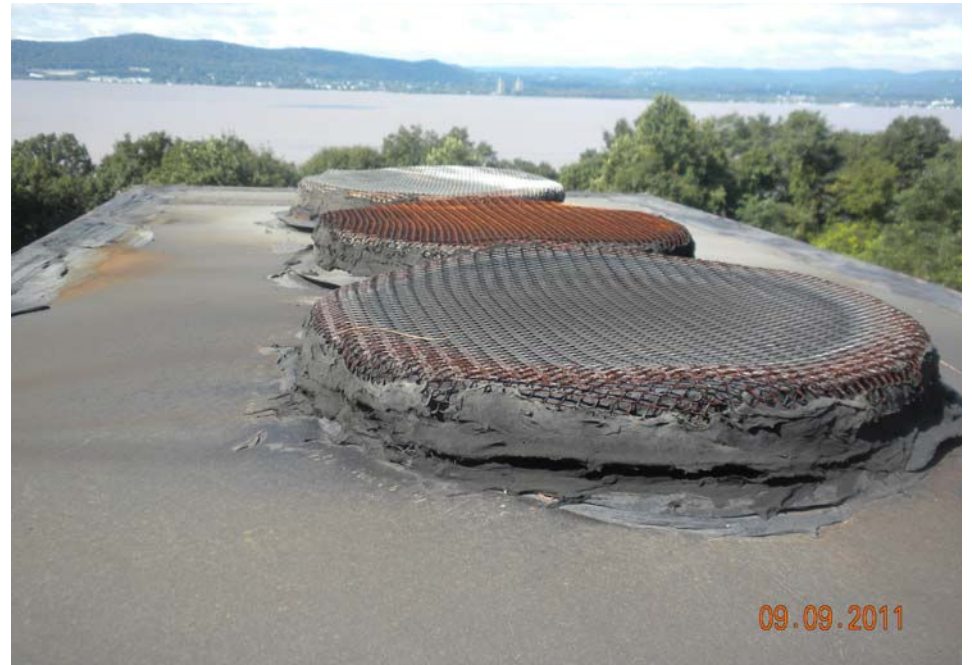
Open joint at chimney flues
