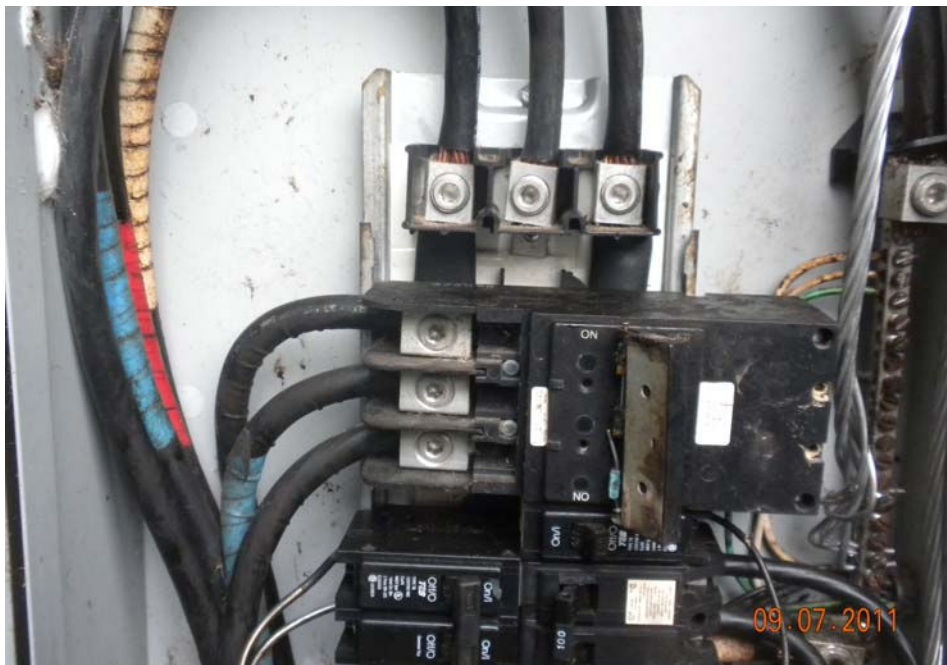
4 wire, 3 phase service
