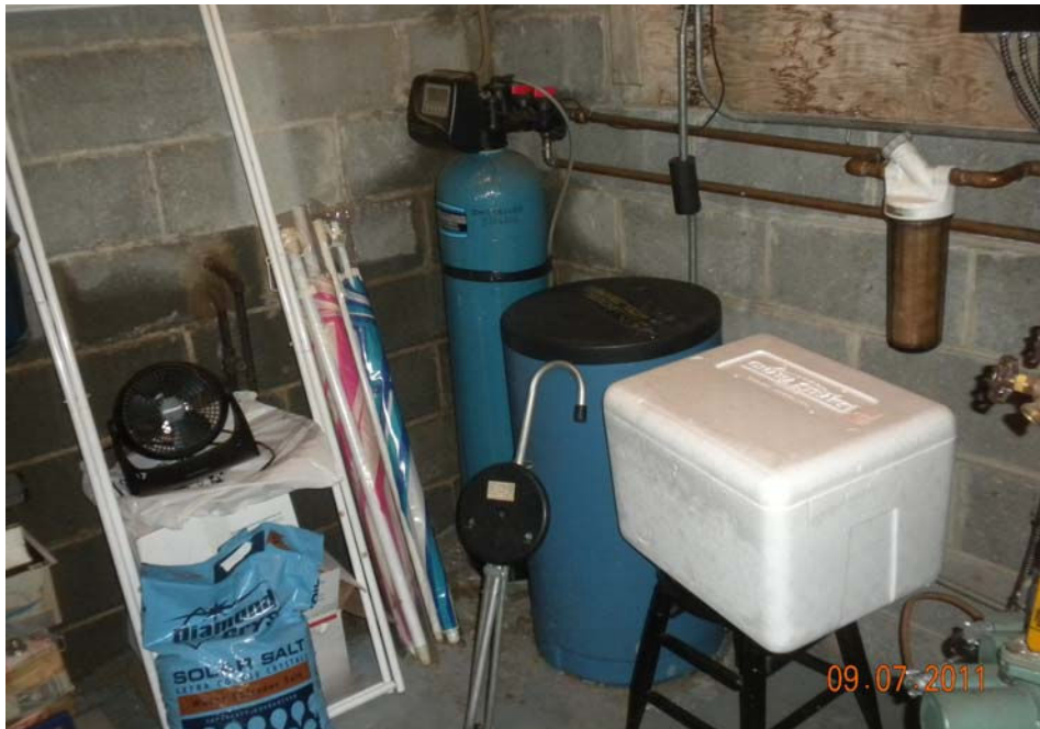
Water softener at main house
