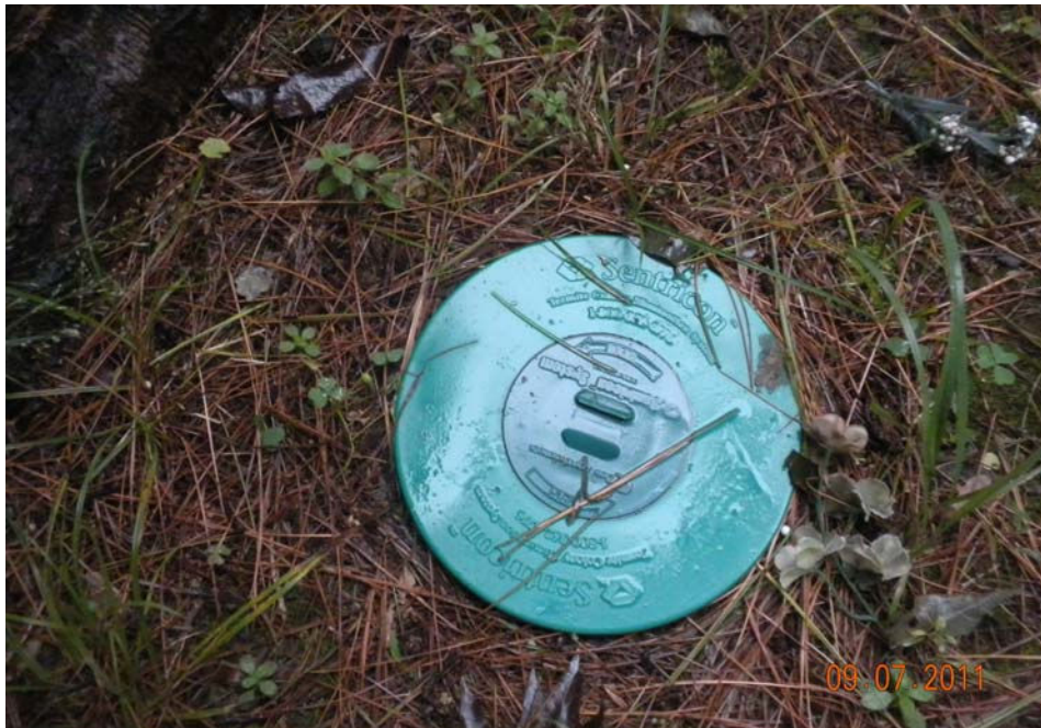
Termite treatment at perimeter of main house
