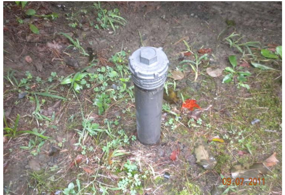
Oil tank fill pipe at the north side of main house
