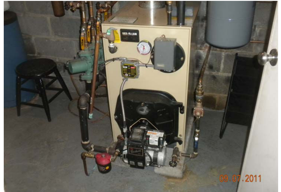
Boiler for main house
