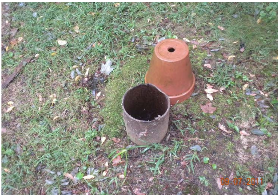
Open well casing needs to be sealed
