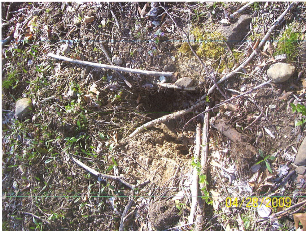
Hole in Embankment
