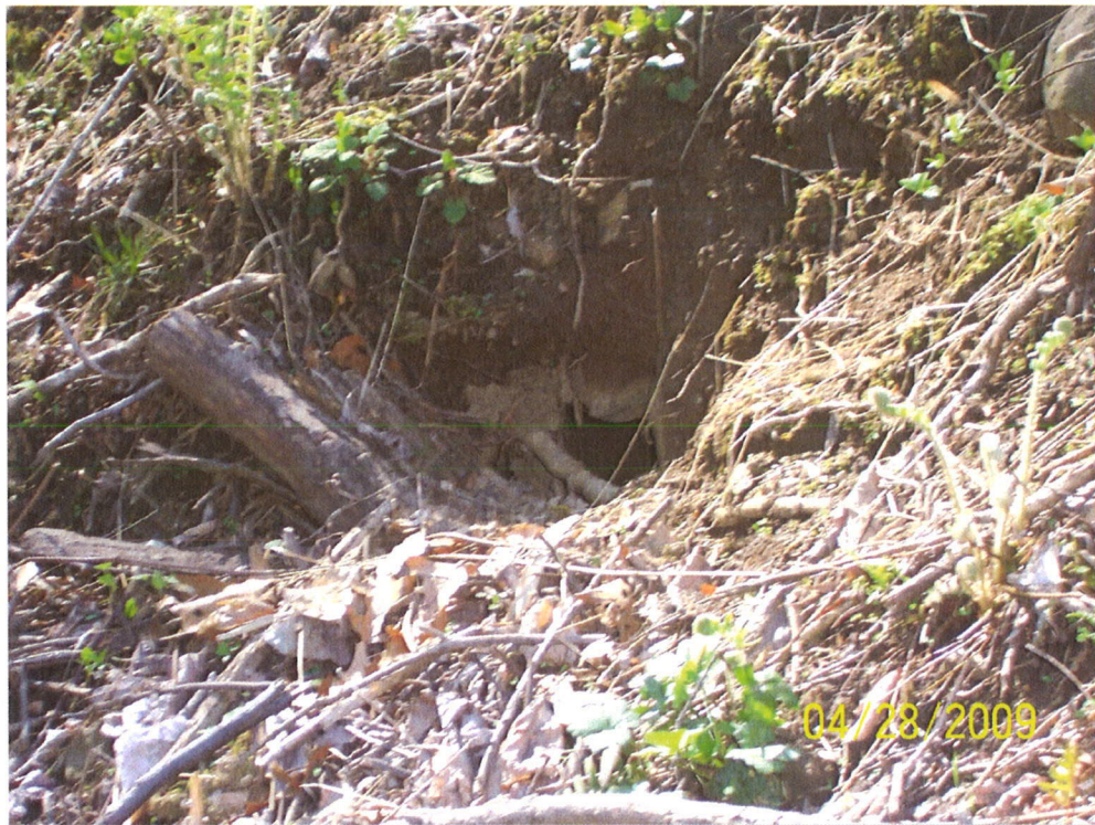
Hole in Embankment
