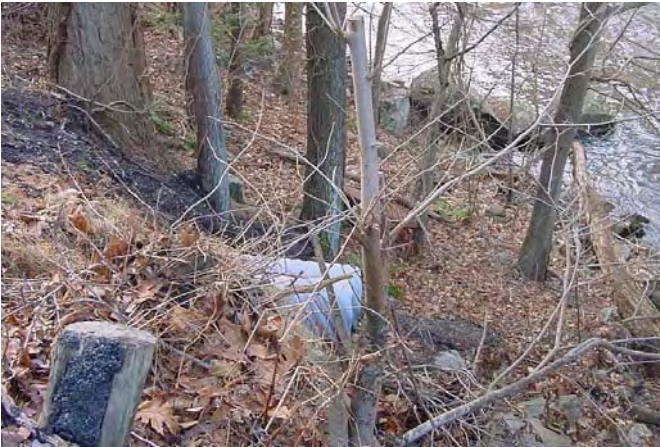
Figure 3-7. Untreated outfalls leading to Croton River.
