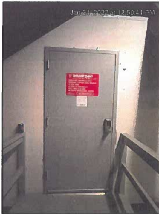
Access to T-Mobile Equipment
