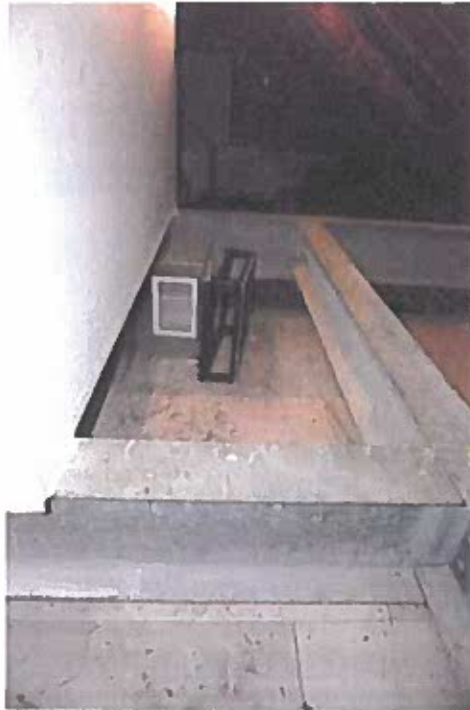
Photo 7: T-Mobile Steel Equipment Platform In Attic
