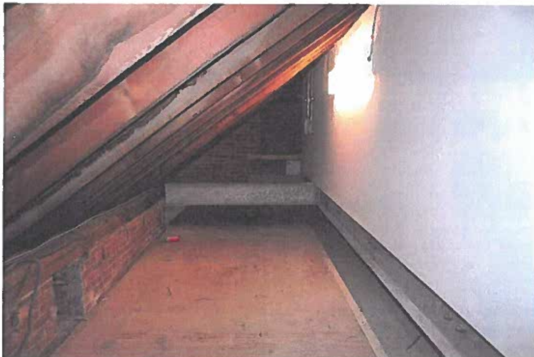
Photo 6: T-Mobile Equipment Shelter in Attic
