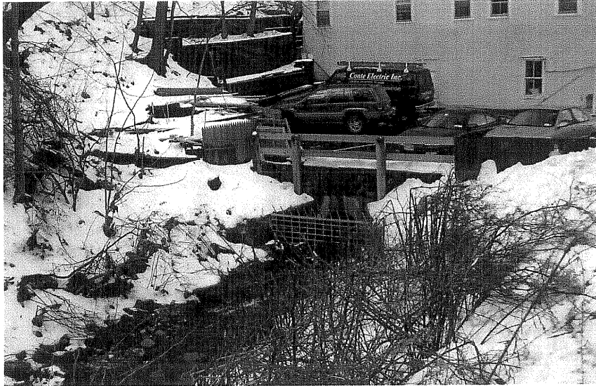
Inlet at Lot 30 on Brook Street
