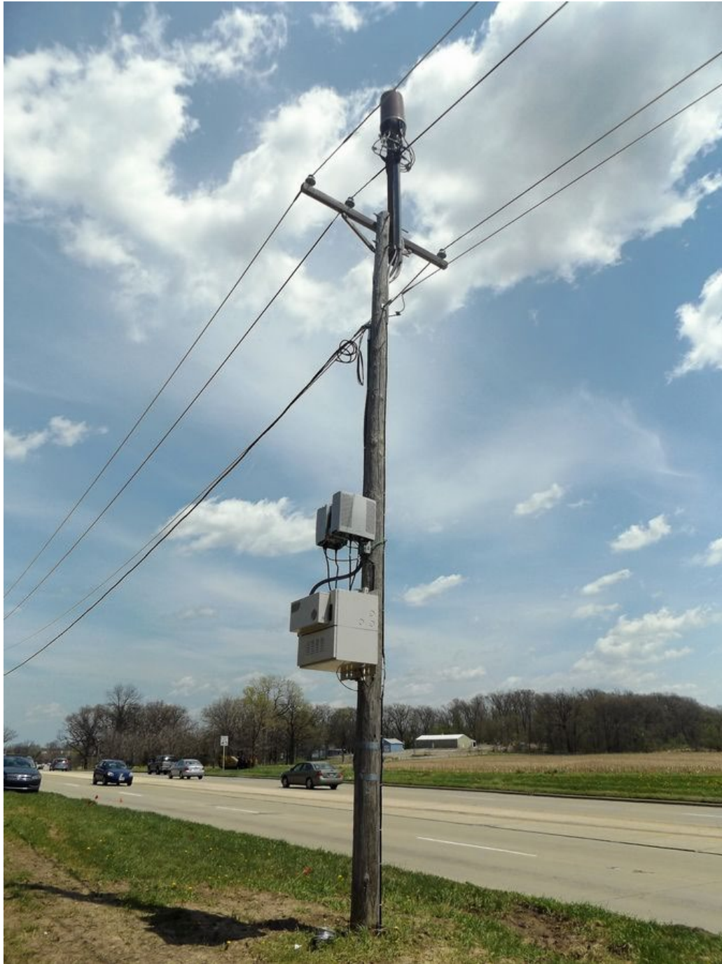
Small Wireless Facility: Utility pole installation with pole-mounted equipment cabinet and pole-top extension.
