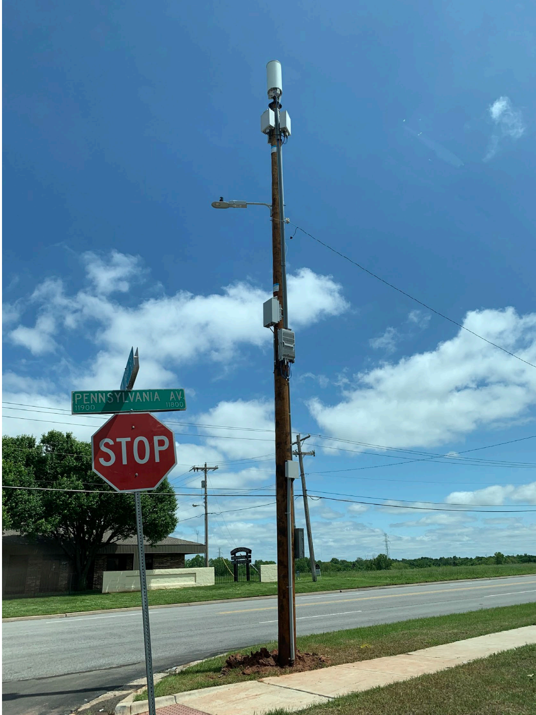
Small Wireless Facility: Utility pole installation with pole-top antenna and pole-mounted equipment.
