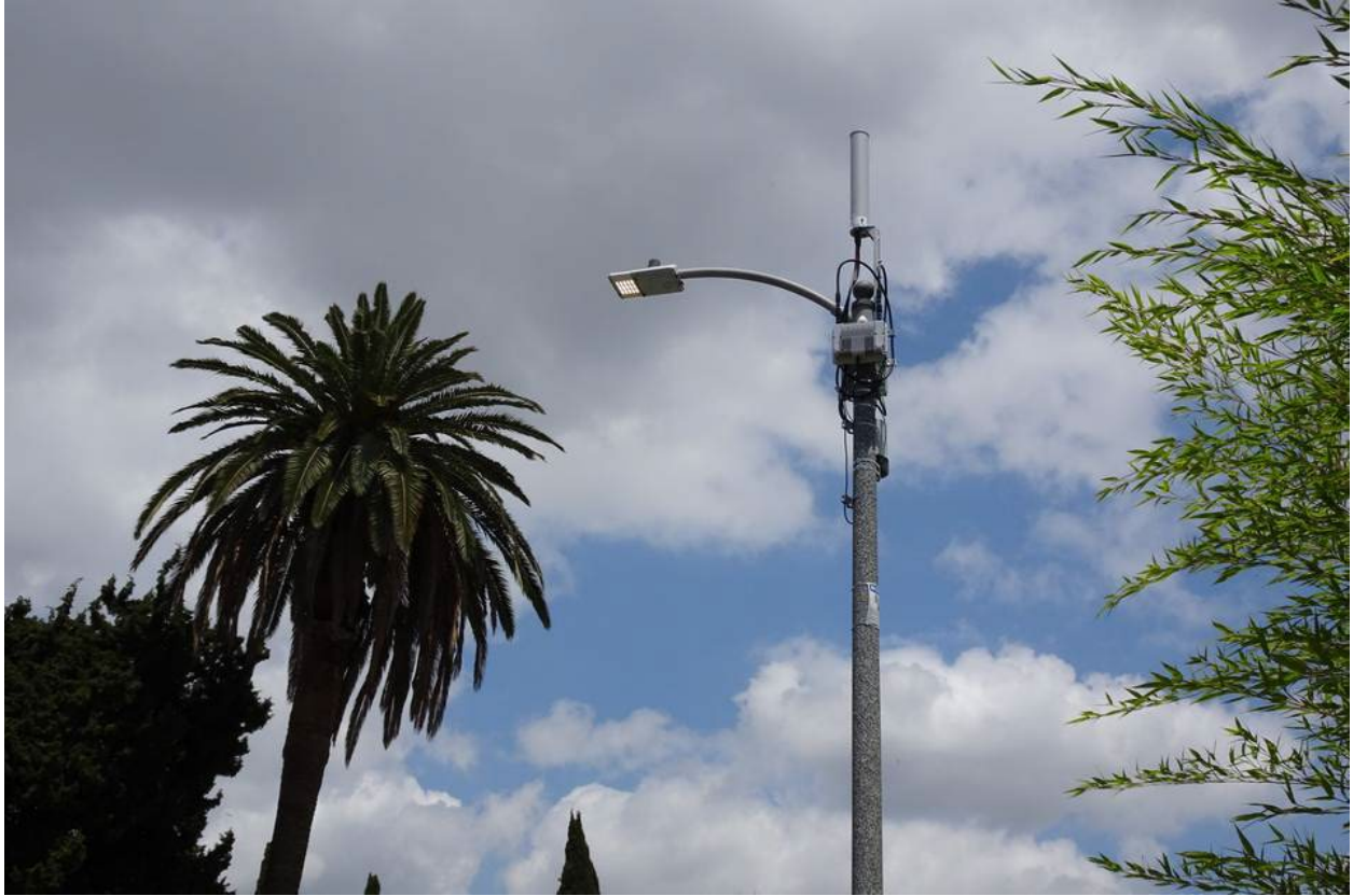
Small Wireless Facility: Streetlight installation with pole-top extension and pole-mounted equipment.
