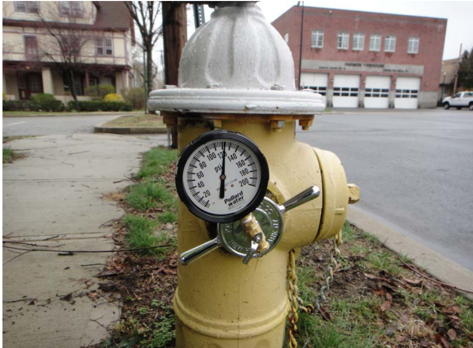
Hydrant B (Wayne St.): Static pressure of 122 psi.
