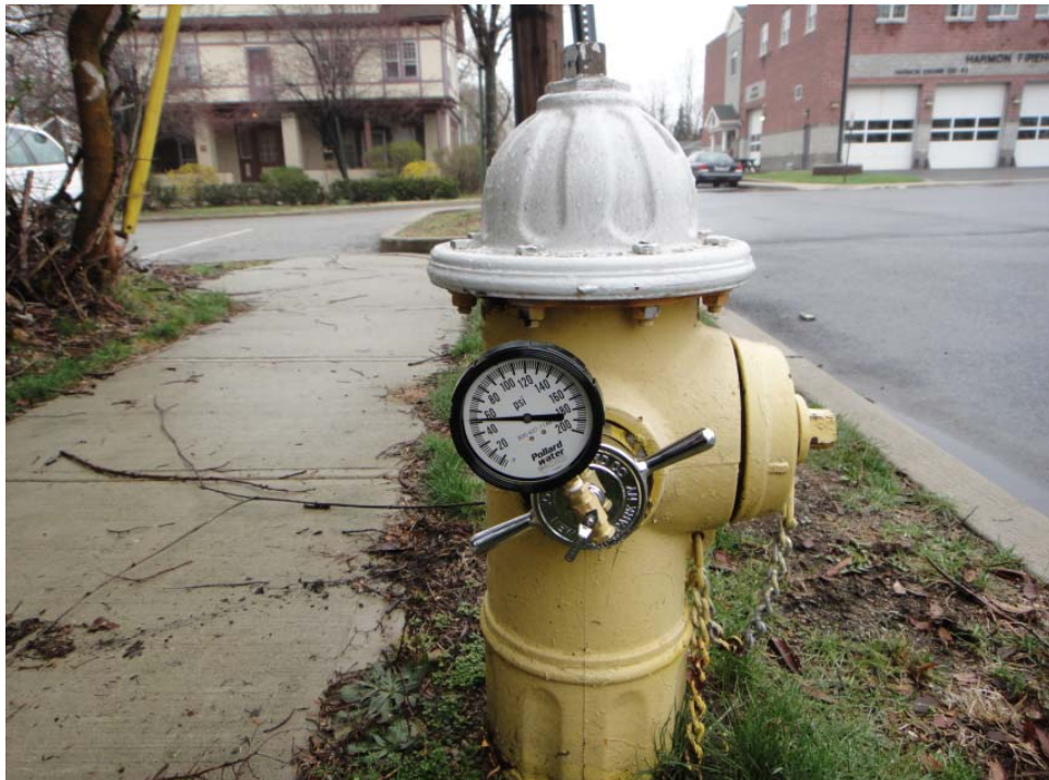
Hydrant B (Wayne St.): Residual pressure of 53 psi.
