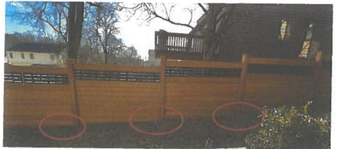
Panels partially buried when possible to minimize step-up impact
