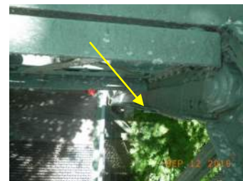
Truss diagonal bowed due to overstress (right of photo)
