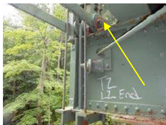
Missing nut on bottom chord. Also shows retrofit attachment to floorbeams
