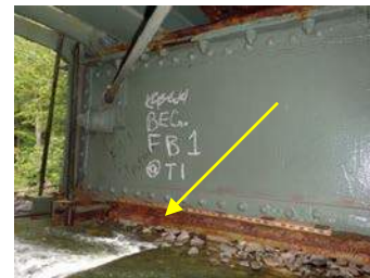
Cracked cover plate weld
