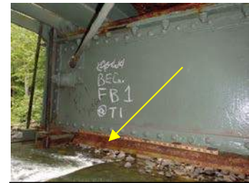
Cracked cover plate weld
