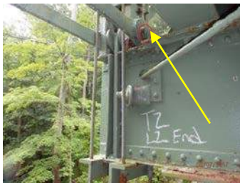
Missing nut on bottom chord. Also shows retrofit attachment to floorbeams
