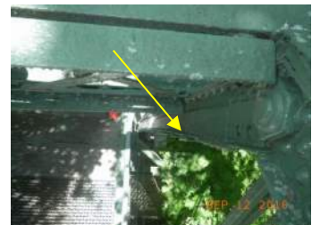
Truss diagonal bowed due to overstress (right of photo)
