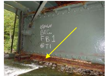
Cracked cover plate weld
