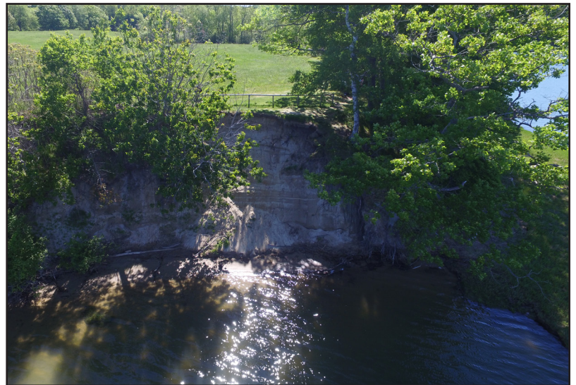
Photo above shows erosion at Maine Audubon Gisland Farms. Maine Geological Survey has been monitoring this site to assess the change in erosion over several years. Photo Credit: GPCOG
