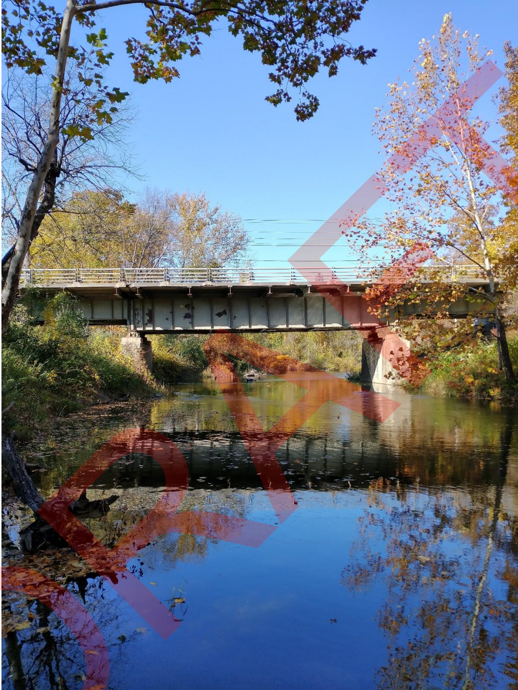
A bridge over the Normanskill on State Route 146 near Tawasentha Park. Bridges like this one may need to be re-engineered to properly accommodate cycling/pedestrian users as well as vehicles.
