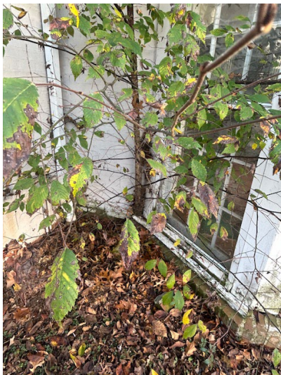
Exterior Vegetation Damage
