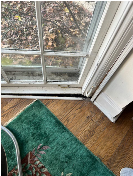
Interior Floor Vegetation Damage
