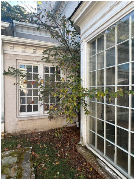
Exterior Vegetation Damage
