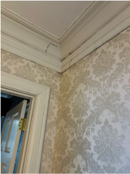
Interior Water Damage
