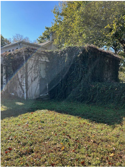
Exterior Vegetation Damage
