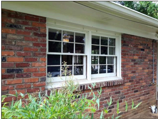
2.3 Item 5 (Picture) Missing Storm Windows
