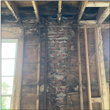
water damage @ rear wall
