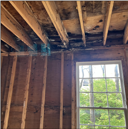
water damage @ master bedroom wall
