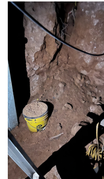
Basement Crawl - Foundation/Hardpack Erosion.
