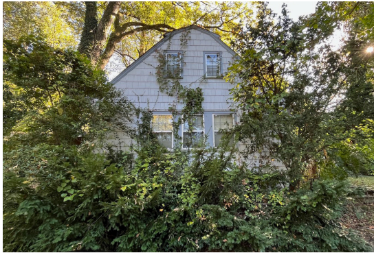
North Elevation - Facing Webster Lane - Overgrowth, Vine Intrusion.
