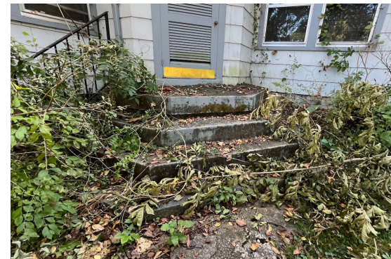
Existing Front Porch - Concrete Step Long-Term Settlement.
