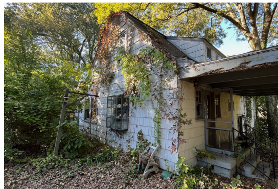
South Elevation - Rot at Carport, Siding, Trim, Vine Intrusion.
