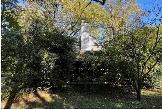
West Elevation - Overgrowth.
