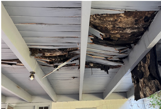
East Elevation Area - Carport Roof Structure Failure/Deterioration.
