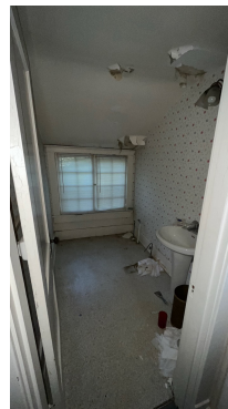
Ceiling Leak Damage - Upper Floor Bath
