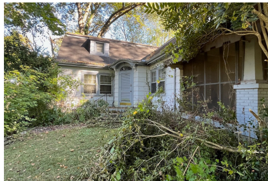
Northwest Elevation - Vine Intrusion, Exterior Deterioration.
