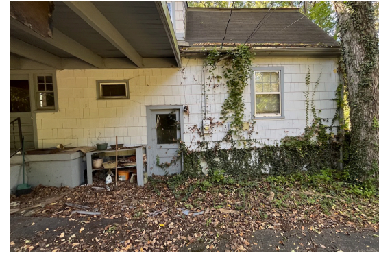
Partial East Elevation - Vine Intrusion, Finish Deterioration.
