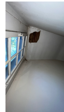
Celing Leak at Stair - Upper level.
