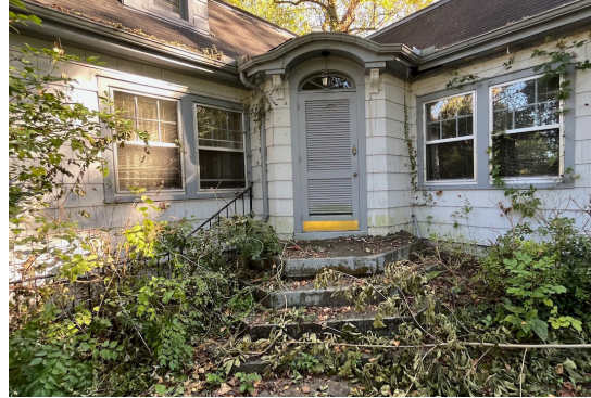
Front Entrance Elevation - Vine Intrusion, Settling, Rot.
