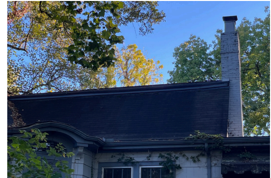
Roof Framing Deflection.
