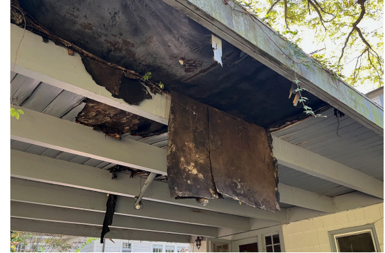
East Elevation Area - Carport Roof Structure Failure/Deterioration.
