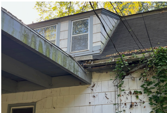
East Elevation Detail - Rot, Vine Intrusion, Water Intrusion at Dormer.
