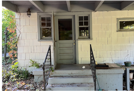
Partial East Elevation - Settlement of Stoop.
