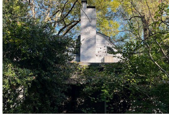
West Elevation Detail - Rot, Overgrowth.
