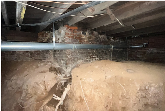
Fireplace/Chimney Footing Erosion/Settlement.
