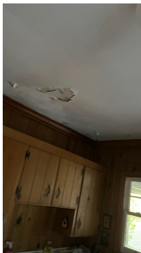
Water Leak Damage - Kitchen on Main Floor
