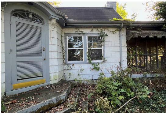
Northwest Elevation Detail - Vine Intrusion Removed Paritally, Deteriorating Finishes, Screen Framing.
