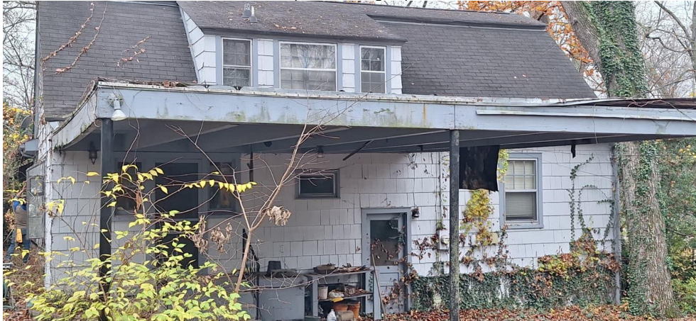
CARPORT – NOT HISTORIC (But damaged)
