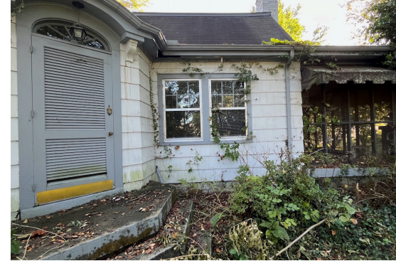
Existing Front Porch - Vine Intrusion Removed Partially, Wood Rot.
