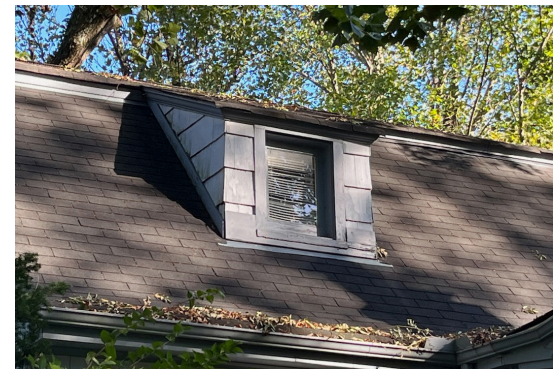
North Elevation Dormer Deterioration.
