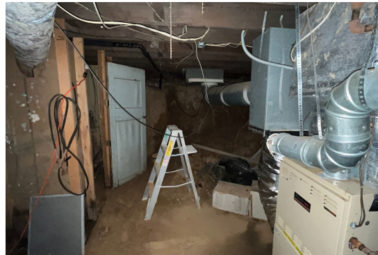
Basement/Crawl - Flooding Sediment.
