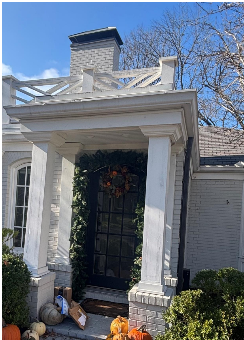
OUT OF PROPORTION AND ROTTING COLUMNS
