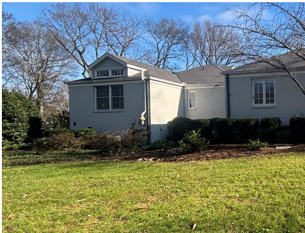
POORLY DESIGNED DORMERS AND CORNICES
