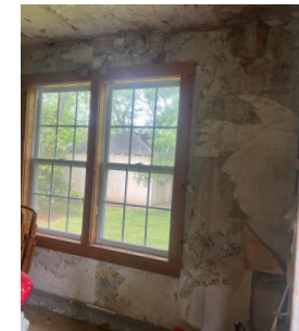
Damage at walls
