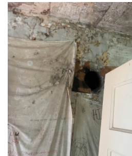
Hole at interior
