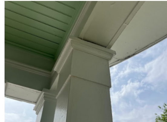
Exterior Damage at Porch
