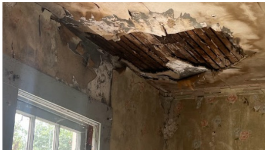
Damage at ceiling
