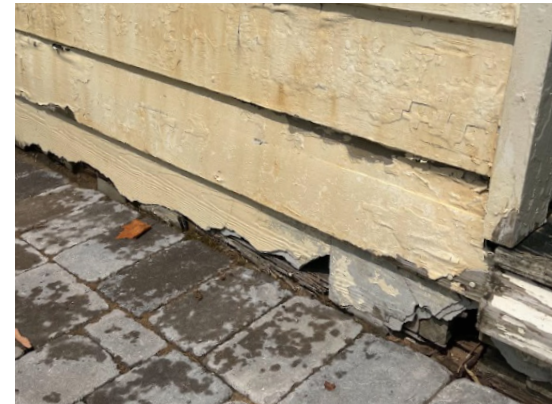
Damage at exterior siding
