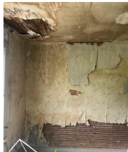
Damage at walls and ceiling
