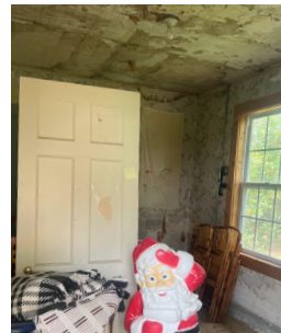
Damage at walls and ceiling
