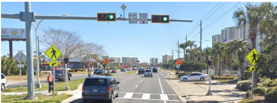
MIDBLOCK TRAFFIC CONTROL SIGNAL
