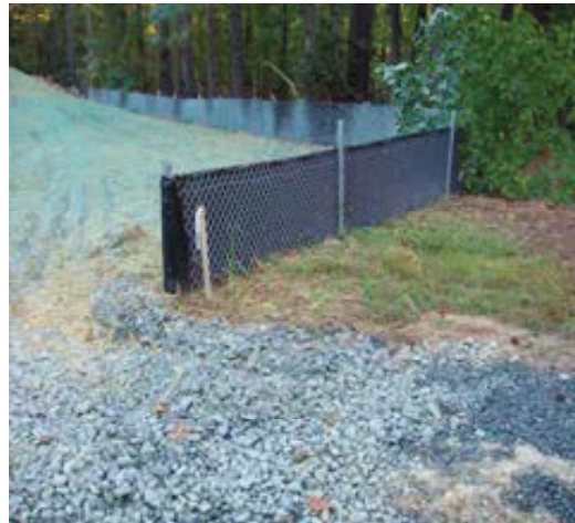
Super Silt Fence
