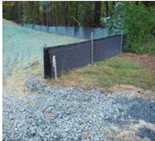
Super Silt Fence
