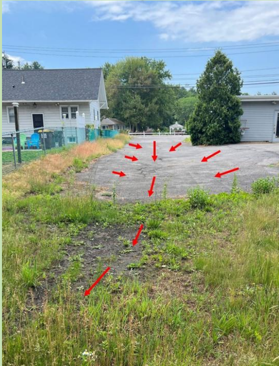
Arrows show direction of drainage. Lawn area is where retention basin is proposed.
