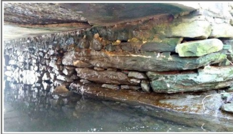
Large stones in the abutments beneath the Kings Highway North Bridge may be remnants of a much earlier bridge. (Photo/Wendy Crowther)
